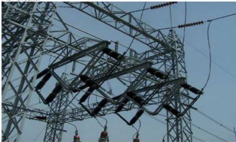
Pic 2 disconnect switches 102 and 106
