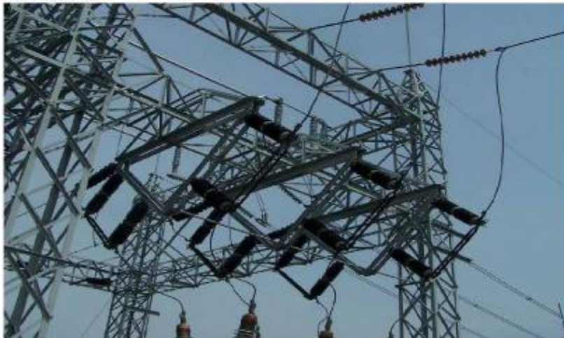
Pic 2 disconnect switches 102 and 106
