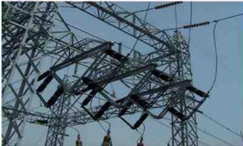
Pic 2 disconnect switches 102 and 106
